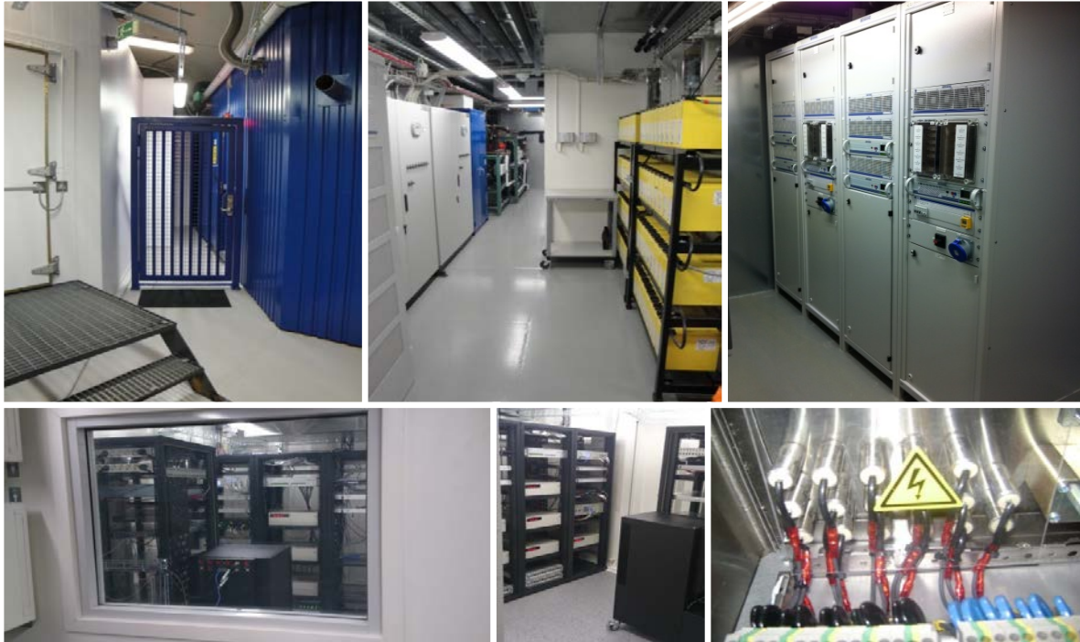
Figure 1: RISE underground clock facility in Stockholm. Upper left picture presents the front wall of EMP protected building inside the cavern and the picture below presents a view of the inside of the underground plant with two identical time and frequency laboratories, separated by a wall with a window, both equipped with same amount of clocks, GNSS receiver and other timing instruments. The upper middle picture presents the outer compartment used for supply systems like climate and power. Electrical power is connected through shielded ducts and metallic leads penetrating the EM-shield are equipped with filters. (lower right picture). Each lab (lower left and lower middle picture) is climate regulated by redundant coolers and a central dehumidifier. DC UPS systems for distribution of 24V and 48V with battery capacities for > 1 hour of sustaining the operation of vital equipment (upper right picture).
