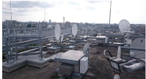
Fig. 7. The rooftop of the NICT building. Two platforms for MWL GT and some TWSTFT antennas are seen.
