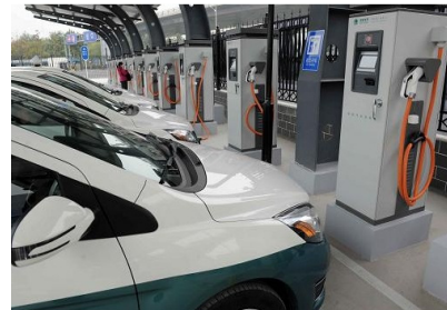
Figure 2. The Electric vehicle (EV) charging facilities
