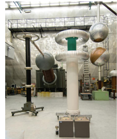
Capacitive divider Tettex up to 400 kV
