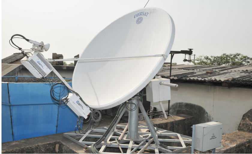
Fig. 10: Antenna unit of TWSTFT system installed on terrace of main building of NPLI.
