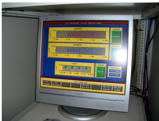
Figure 3 Status display of the automatic switch system
