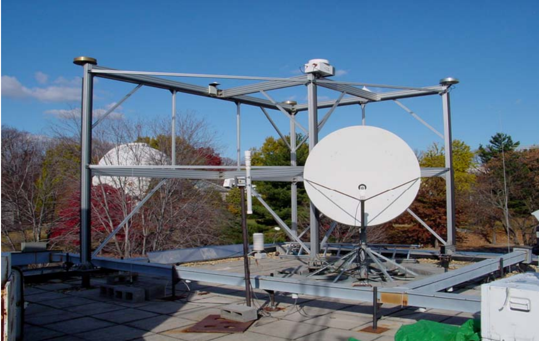
Figure 7. GPS antenna mount, now operational for GPS monitoring, has reduced multipath by roughly a factor of 3. Right of center is a directional antenna used to monitor WAAS signals.
