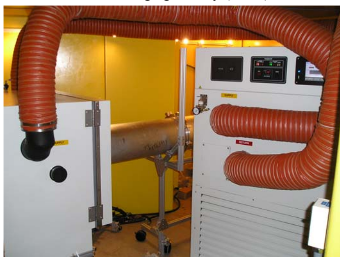
Freeze chamber installed inside BT2.
