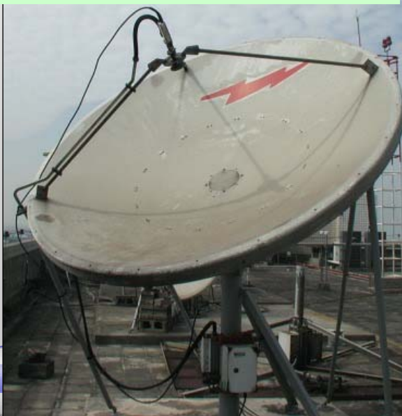
2.4 m antenna (for JCSAT-1B)
