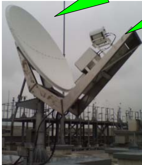
TCE Earth station
