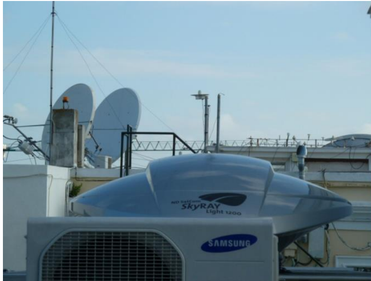
View of the mobile station at ROA
